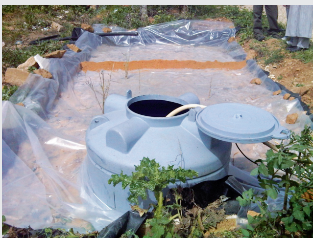
Figure 6: Treatment trench at Jerash, Jordan
